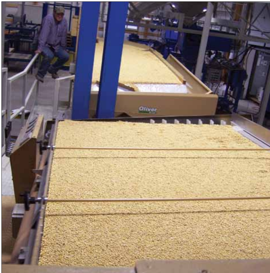
(top) Westrup airstreen. The dust suppression oil tank is in lower-left corner. (above) Oliver gravity separators operating without dust hoods.
