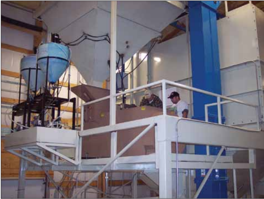
Plant Manager E.W. Browning at the Gustafson seed treater control panel.
